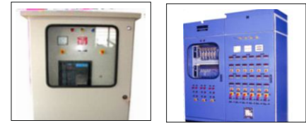
Outdoor Panel Plc Based Panel
