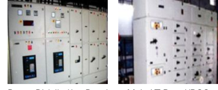
Power Distribution Panel Main LT Panel/PCC
