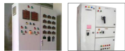
Instrumental Panel Fire Fighting Panel
