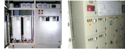
AC/DC Drive Panel MCC Panel
